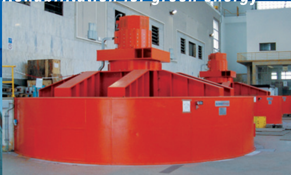
Inside the Chievo power house.
