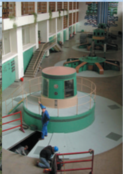
Insight view of Orfeus power house
