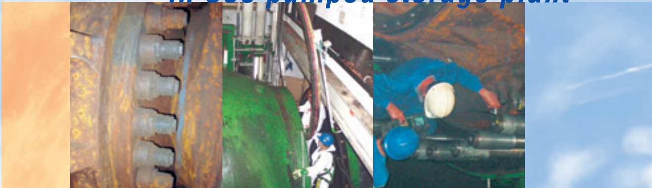
From left to right: Found condition of valve inside Liftout of seal ring Examination of the bolts
