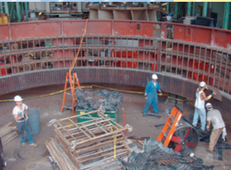
Voith Siemens Hydro's work in progress on the stator repair and rewind at the Robert Moses Plant
